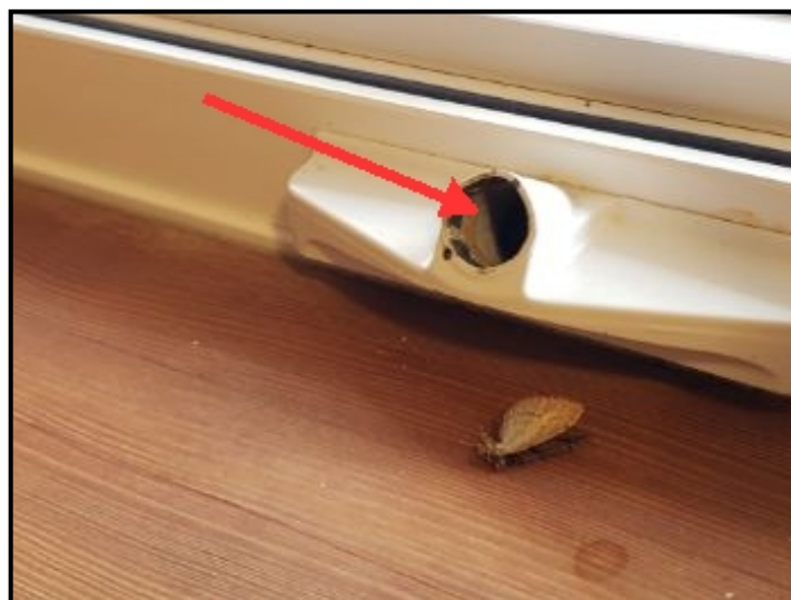
Damaged window hardware upstairs.
