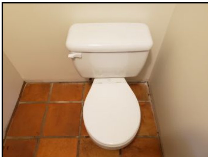
Washroom has loose toilet. Have repaired to prevent future leaking at wax seal.
