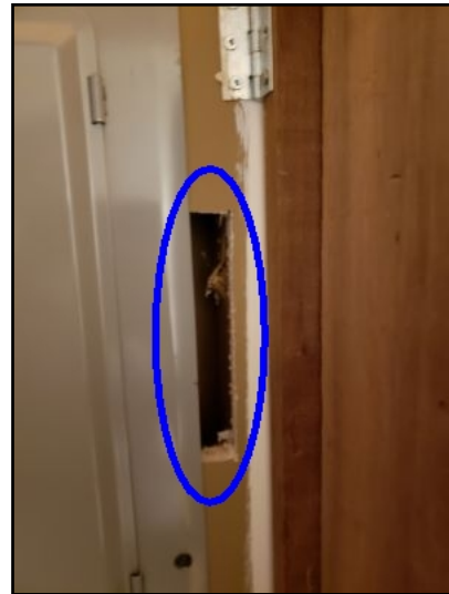
Cover open cut out beside panel for safety.
