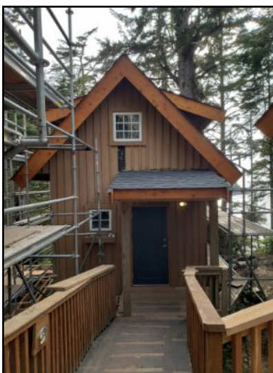
Cedar siding with required building paper noted under siding. Still under construction at time of inspection, almost done.
