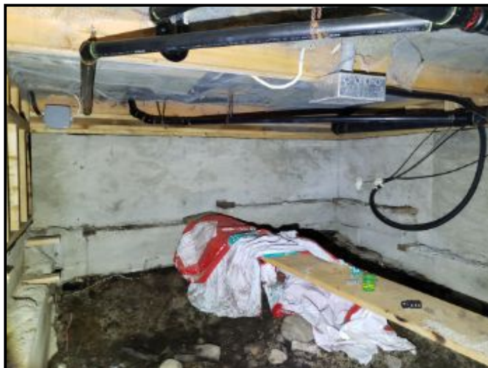
Rodent droppings noted in crawlspace.
