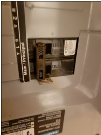
100 amp service with all copper branch wiring.
