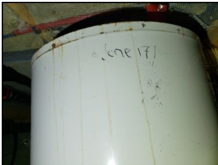
Tank is rusted, damaged and/or leaking. Replacement recommended.
