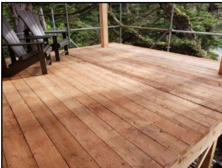
Joist have been constructed, cedar decking is yet to be installed on lower, top deck is complete.
